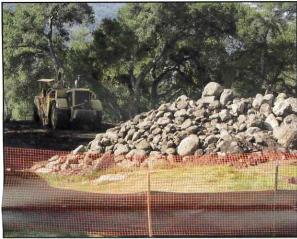
850 truckloads of rocks and boulders such as these had to be removed from the Chapel site.
